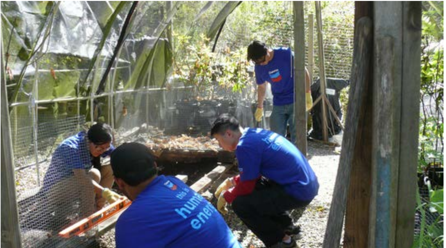
Rebuilding the hoop house benches. The team is leveling the bench supports, which have to be just far enough from truly level for the water to drain out of the channels in the racks.
